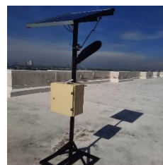
Gambar 3. 14 PJUTS solar Tracking
